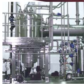
Centritherm used in the wine and beverage processing industries'. Photo courtesy of FT Industrial Pty Ltd.
